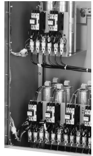
Factory Pre-Wired for Future Expansion
